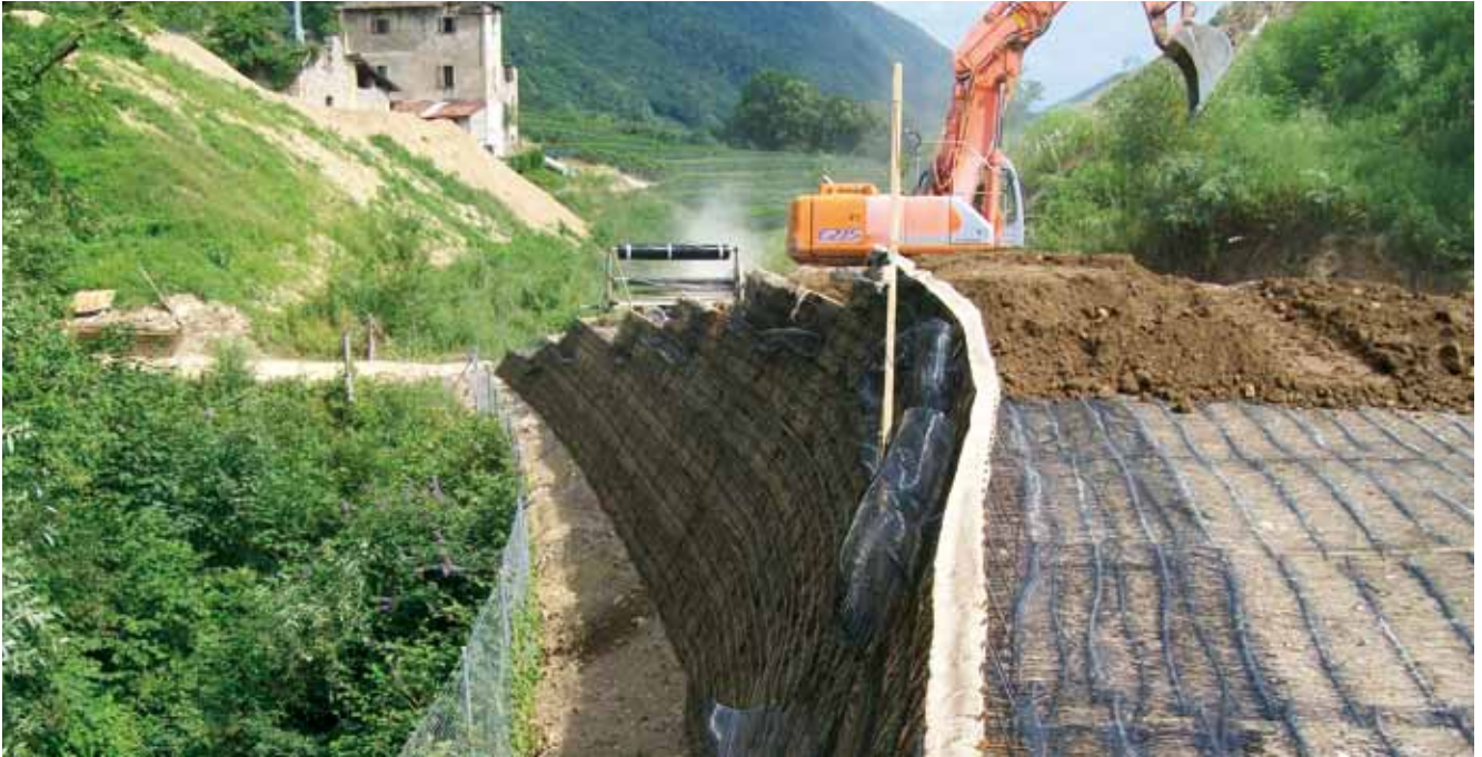
As part of the re-development of the "Castello di Cantone" estate, Switzerland, the inert landfill has been transformed into a terraced hill to create a riding school.
