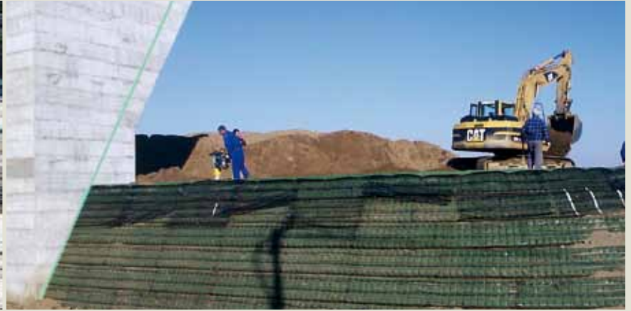
A typical example of a soil reinforced slope adjacent to a concrete structure (e.g. adjoining wing walls or bridge abutments)
