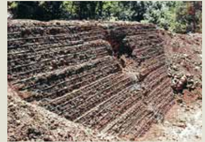
The downhill side of the reinforced rockfall barrier following impact is damaged but remains intact
