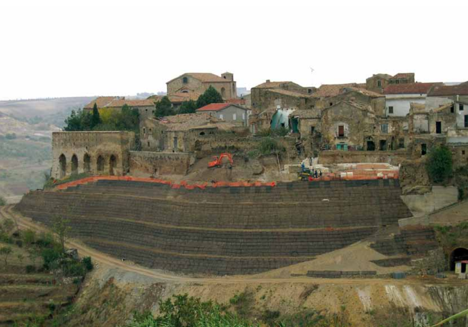
Slope Stabilisation of the historical village of Genzano di Lucania, Italy, in order to preserve the main church and an ancient monastery.
