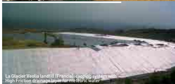
Containment of expanded clay on top of the modified capping system of the Modena Landfill
